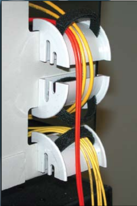
Patch Panel Egress
